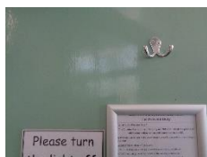
Coat hook too high
